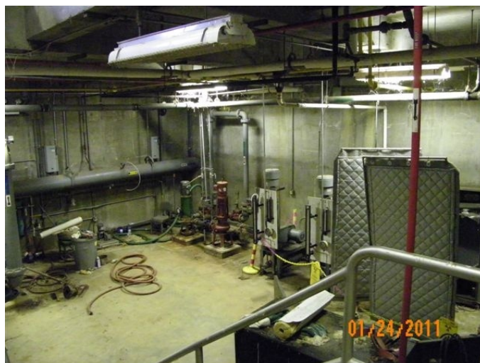
Figure A.101. X-6619 Sewage Treatment Plant Filter Building Radiological Contamination
