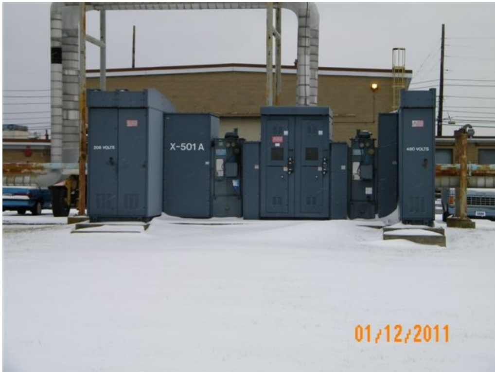
Figure A.104. X-501A Substation
