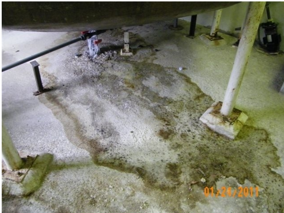
Figure A.172. X-617 Interior Leaks or Spills
