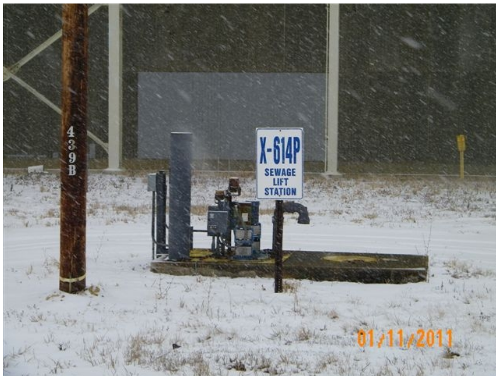
Figure A.90. X-614P North East Sewage Lift Station
