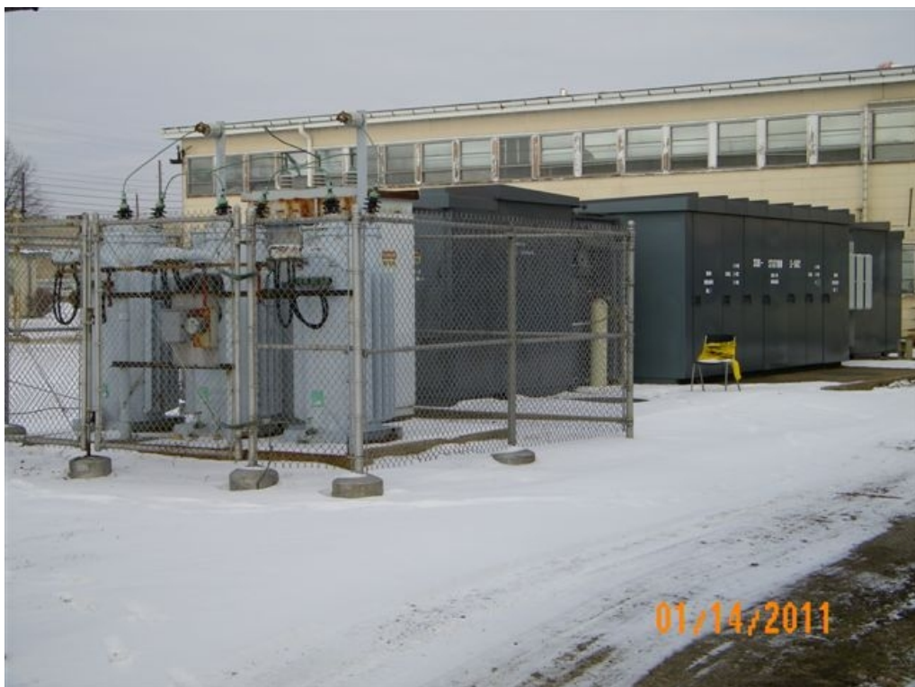
Figure A.105. X-502 Substation
