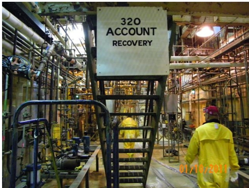
Figure A.26. X-705 Decontamination Building Equipment
