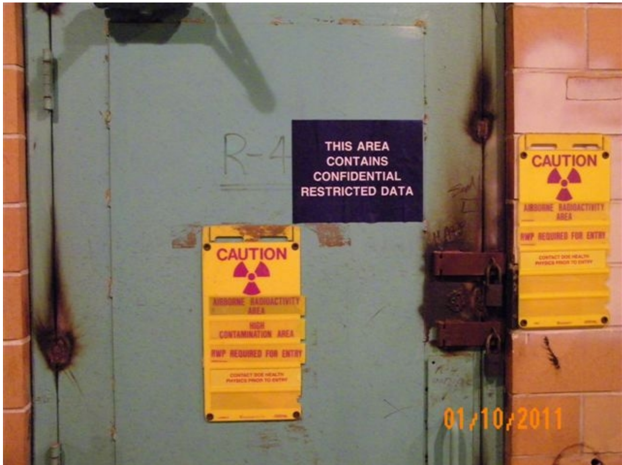
Figure A.29. X-705E Contamination
