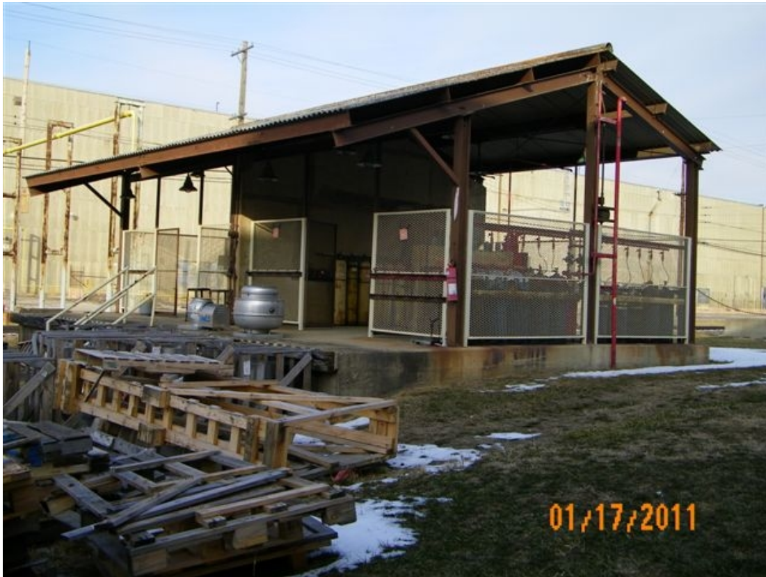
Figure A.33. X-710A Technical Service Gas Manifold Shed
