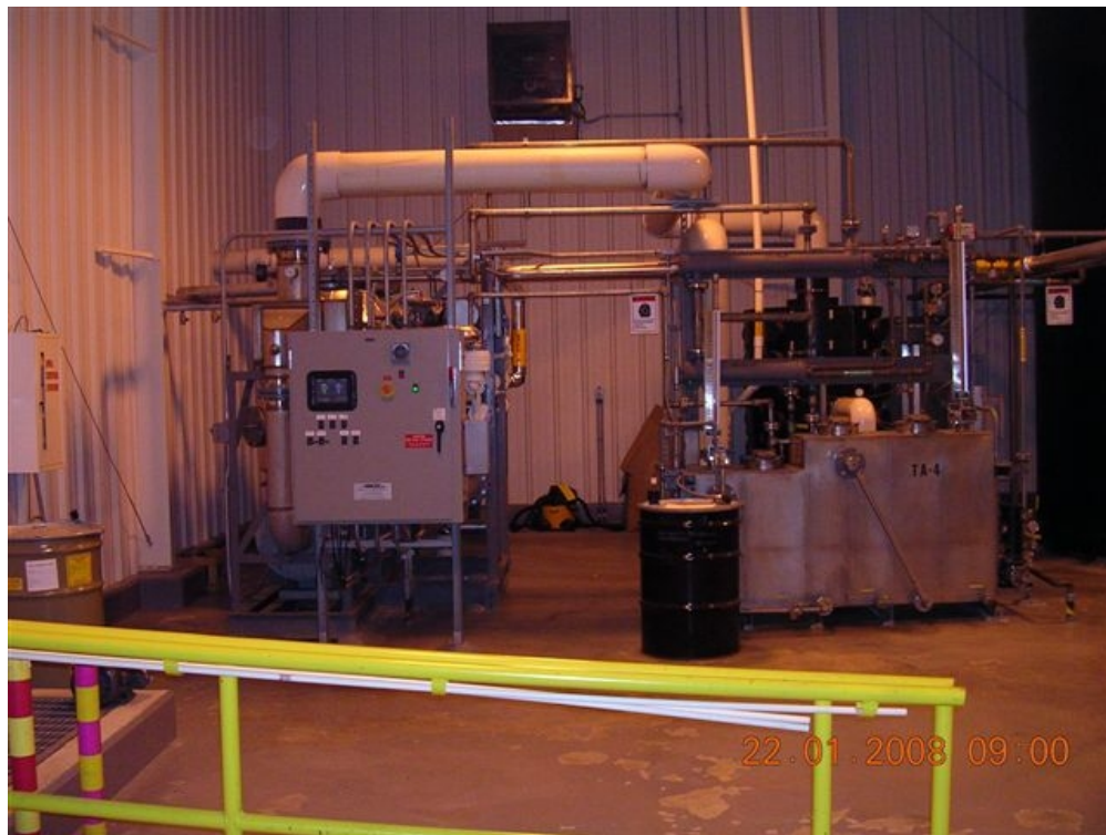
Figure A.181. X-627 Groundwater Pump & Treatment Facility Process Equipment
