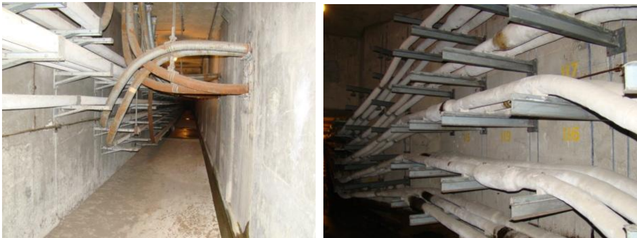
Figure A.106. X-215D Electrical Power Tunnels
