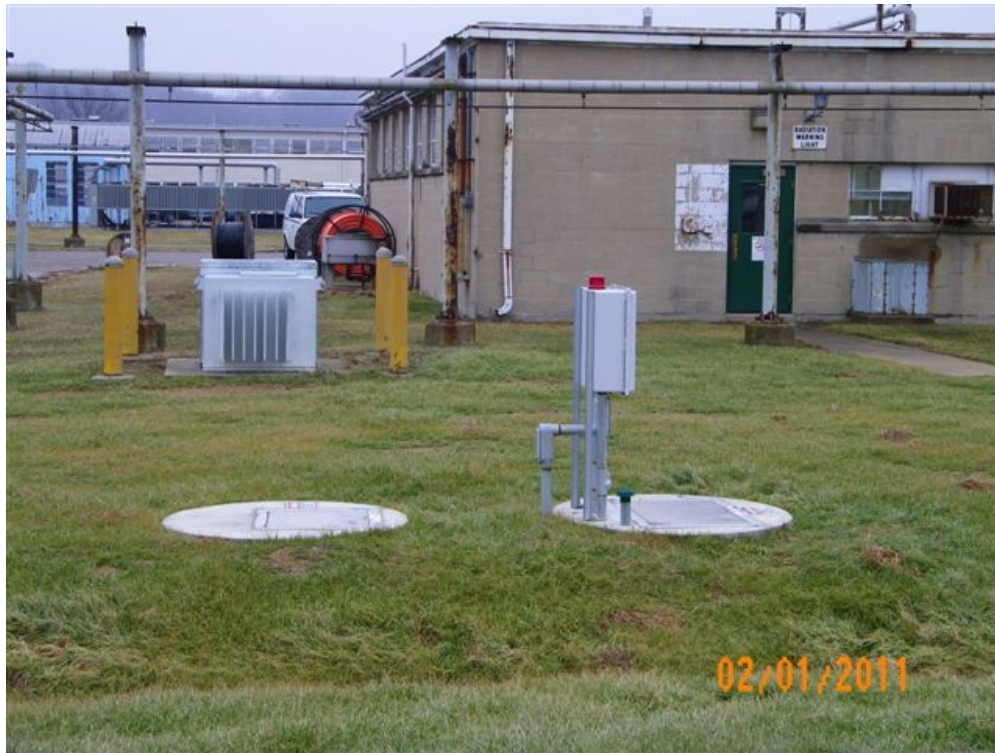
Figure A.91. X-614Q Sewage Booster Pump Station
