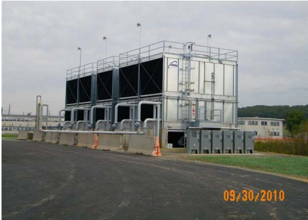
Figure A.110. X-670A Cooling Tower
