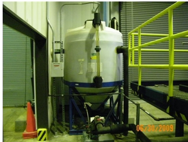
Figure A.175. X-622 South Groundwater Treatment Facility Process Equipment
