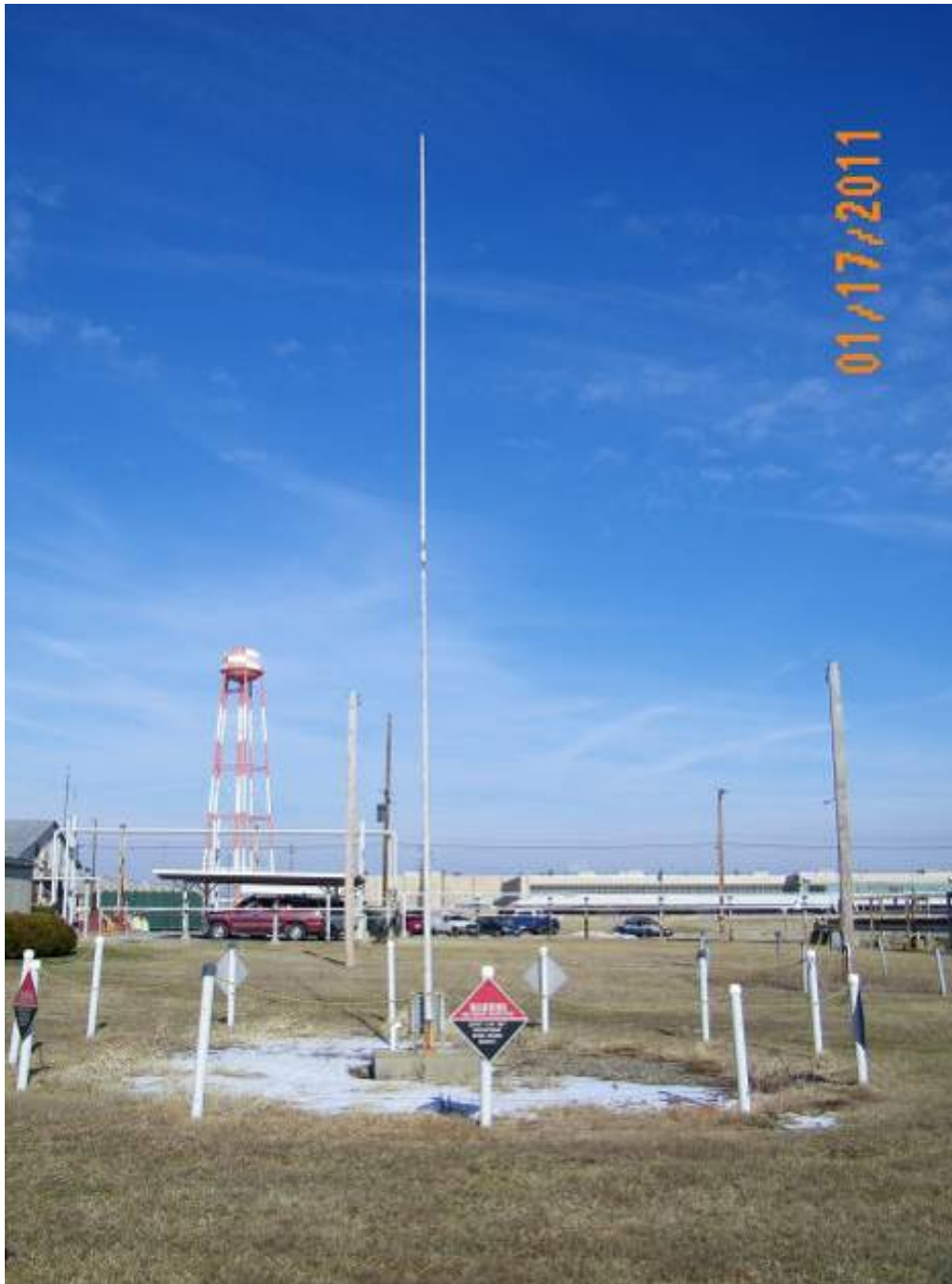
Figure A.62. X-300C Emergency Communications Antenna
