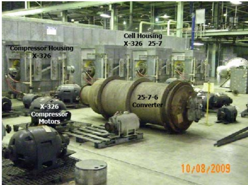
Figure A.11. X-326 Process Equipment
