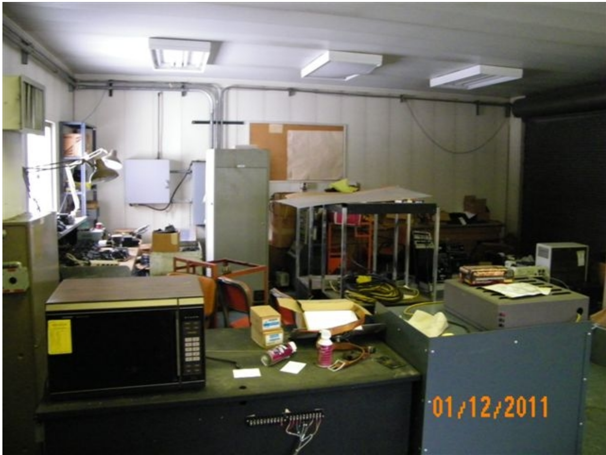
Figure A.41. X-720B Radio Base Station Interior
