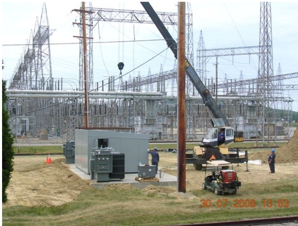
Figure A.107. X-640-1A Substation
