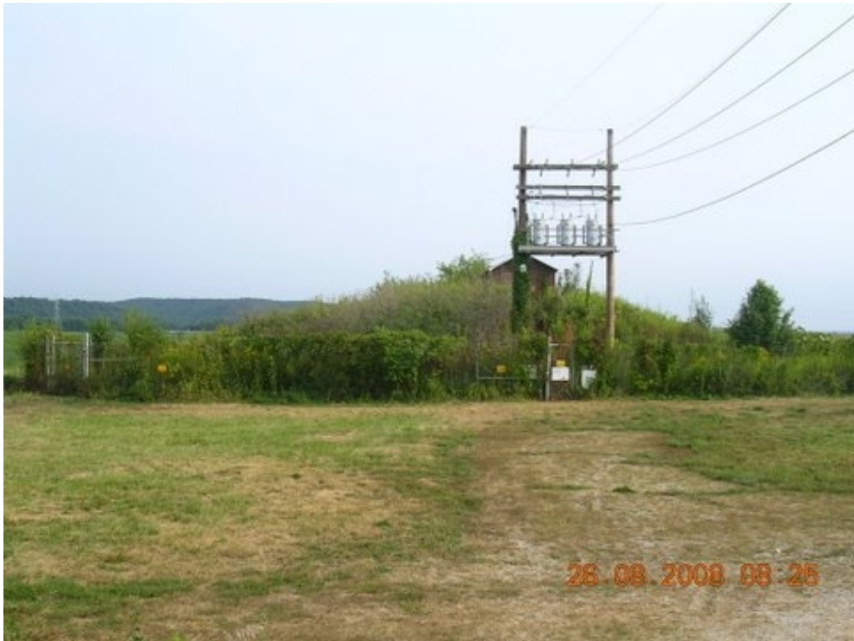
Figure A.77. X-605A [X-605G] Sanitary Water Control House and Transformers Viewed North to South from Well X-605-G3
