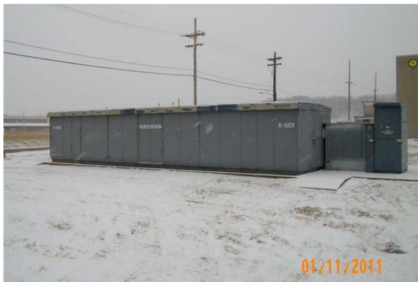
Figure A.103. X-501 Substation
